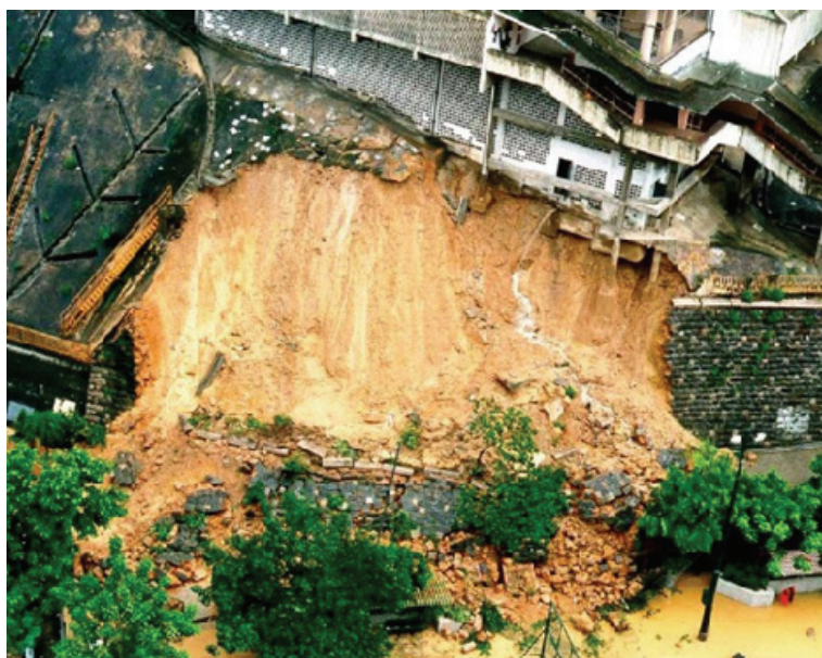
Fig. 1 Landslide at Kwun Lung Lau in 1994 [12]
